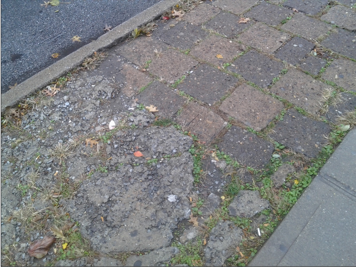
A close-up of the current materials that clog the sidewalk planter spaces along Campus Road. One foot by one-foot concrete tiles and sloppily poured cement are not what these spaces need.
